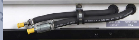
INPUT/OUTPUT FUEL PIPE
